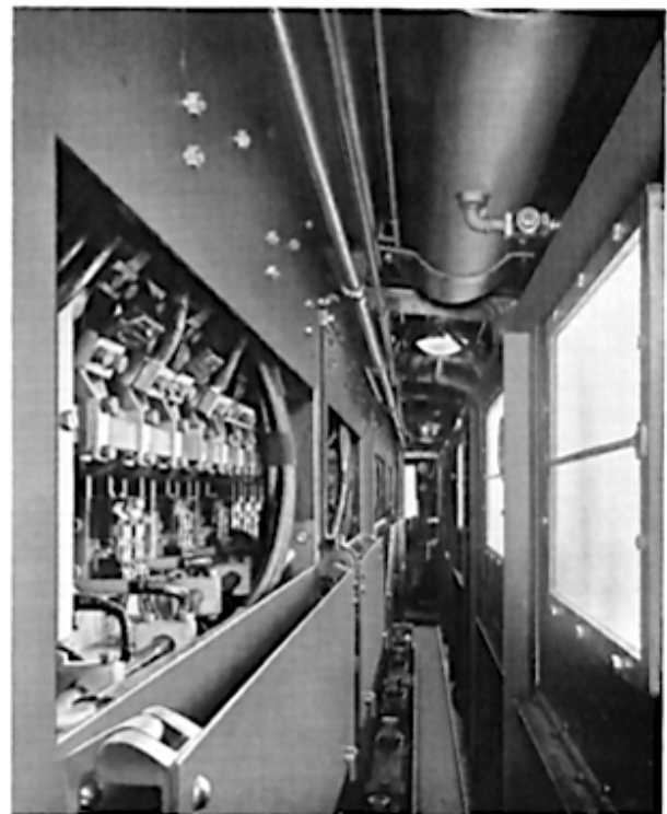
Interior of loco showing walkway between cabs and the access doors open on the banks of contactors
