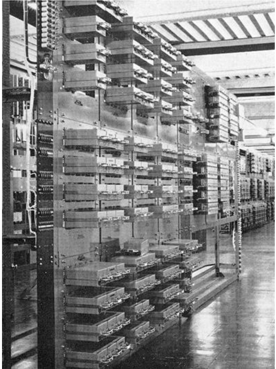
Fig:1 Relay Room in a conventional Signalbox. This technology is being rapidly superseded by solid state, electronic equipment, whilst the lineside equipment is being enhanced with TPWS and ATP systems.
